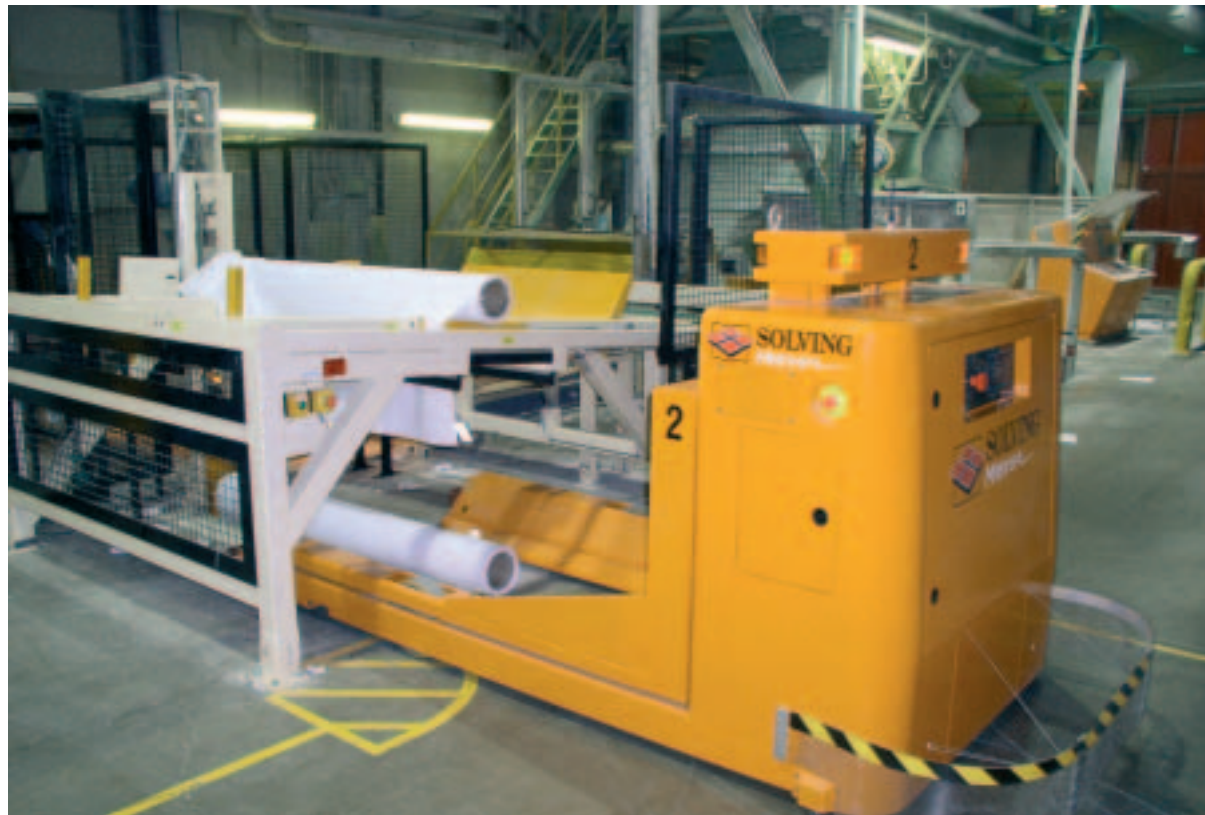
Paper reels are automatically fed to the different stations of the sheet cutter
